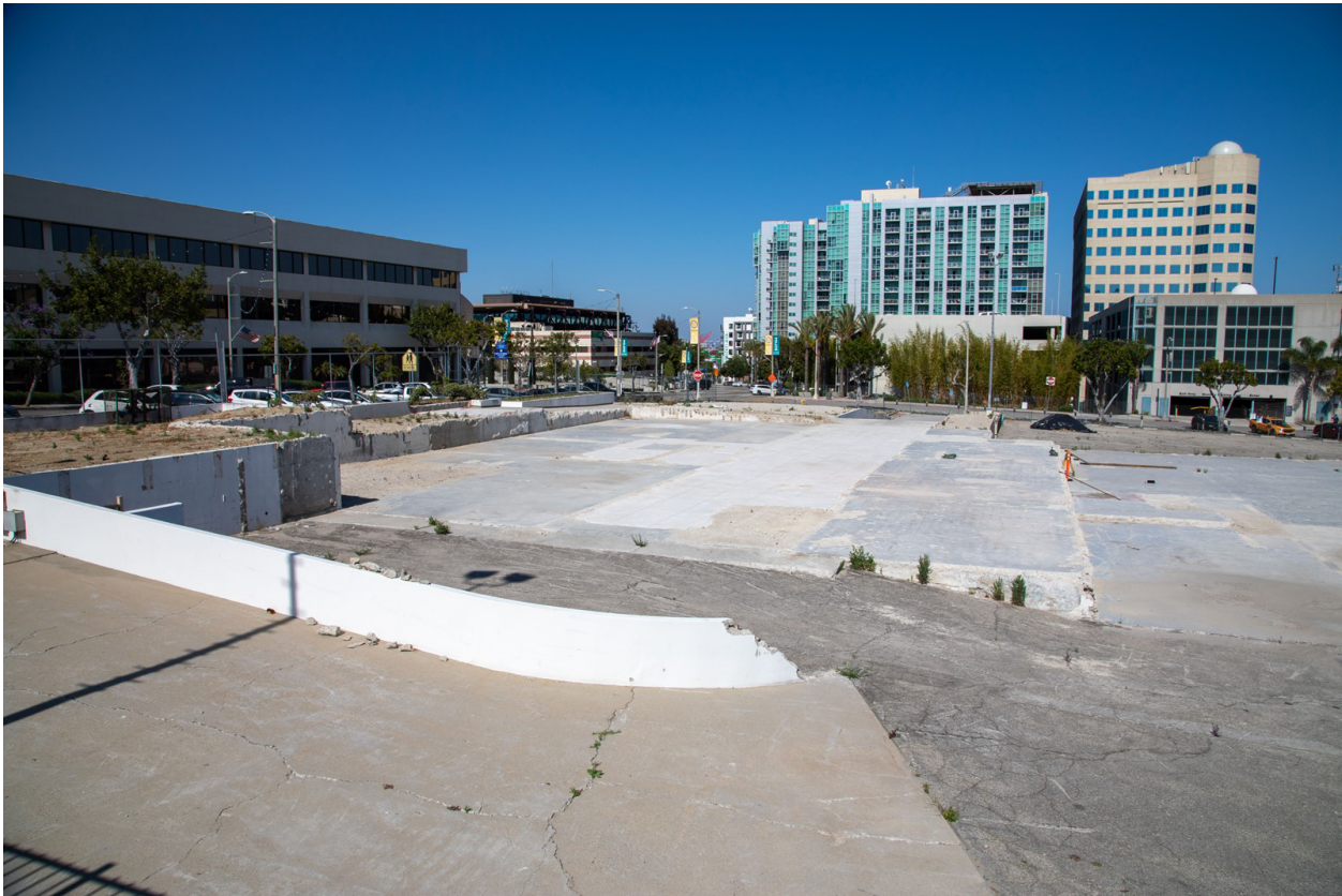
Among the first stages of work on the mixed-use apartment complex at Sixth and Centre streets in San Pedro will be to remove the foundation of the old courthouse and surface parking lots, which have been kept in place to hold down the dust on the cleared site.
